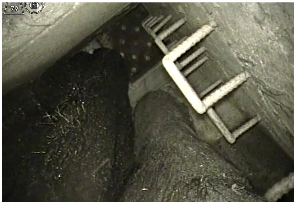
Figure 3 – 600 diameter stormwater pipe – tree root obstruction at Pit 2 (210817 – ALS CCTV Report)
